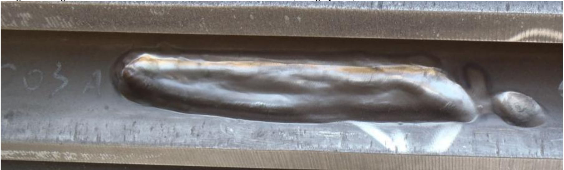
Fig 10 Final profile and surface finish of excavation
