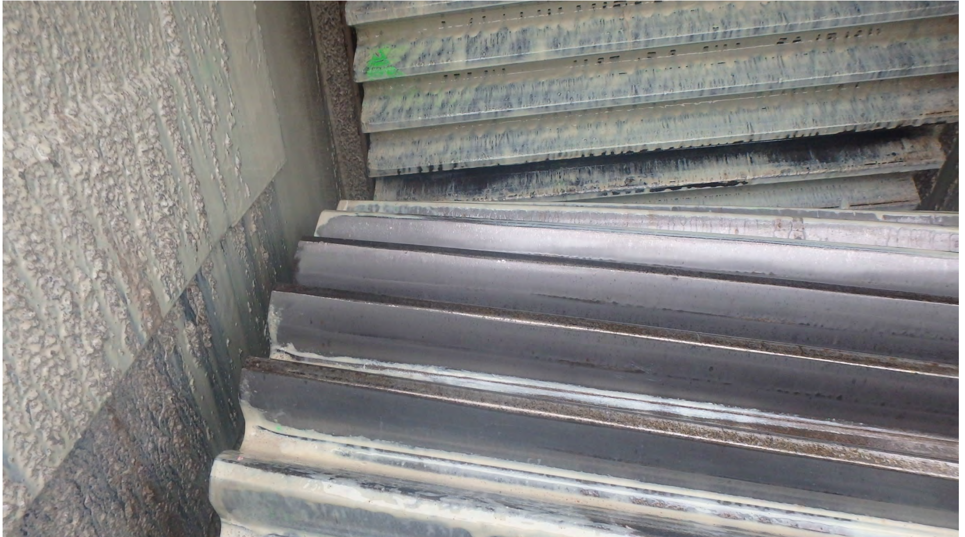
Pinion gear drive end. Note the raised pitch line.
